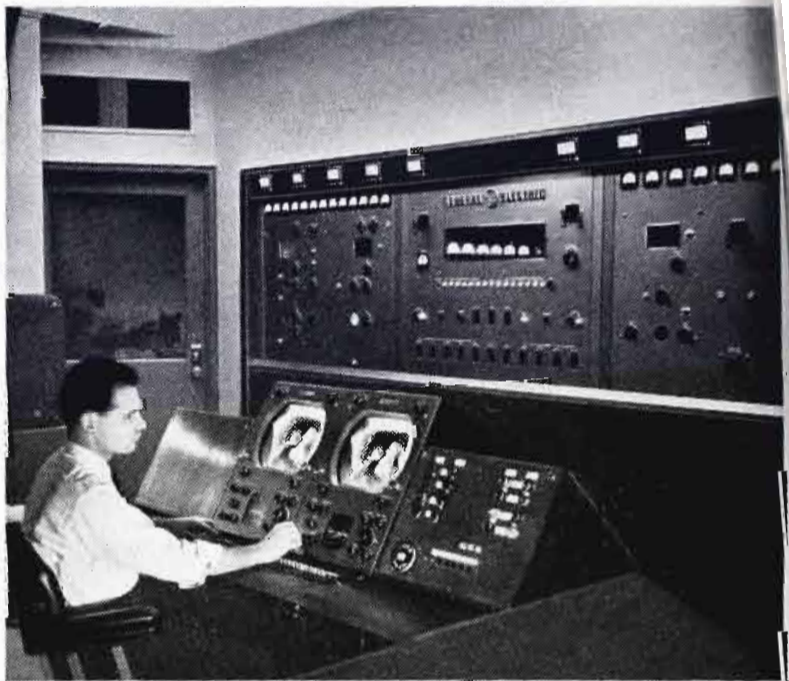
G-E transmitter equipment in CBS-Empire State Building, New York installation.
